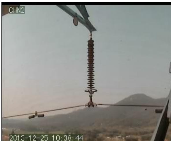
Figure 10. Typical visible image of the insulator obtained from the master station
